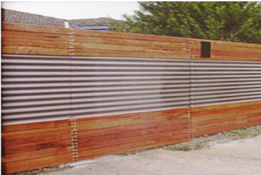
Fencing - Corrugation with Rusted Metals and Wood
